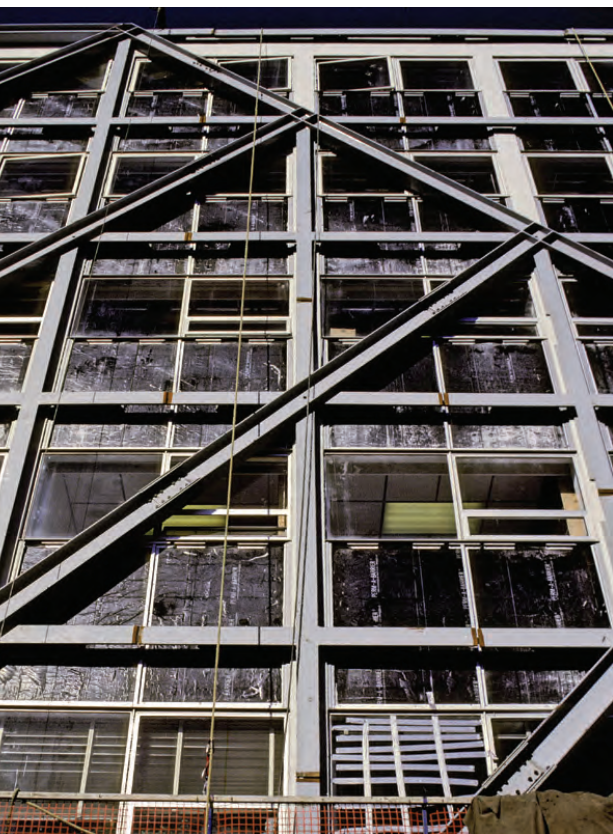
FIGURE 14 Cross Braces Strong, diagonal beams called cross-braces have been installed in this building to improve the structure's ability to withstand seismic waves.
